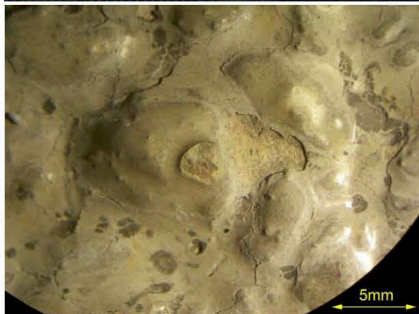
Magnified view of the stack stone rear face showing the glossy fine-grained laitance covering the aggregate grains. The sandy matrix can be seen under the surface layer.
